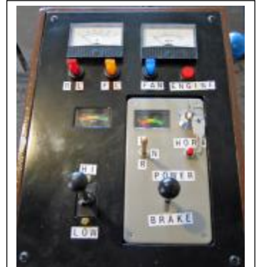
Photo Peter Downes Peter's controller for his Class 73 EDL. The two meters are for the main and auxiliary batteries.
