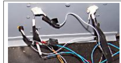
Photo Colin Gross A typical LED lighting installation.
