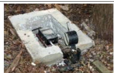
Photo Colin Gross The first of the new concrete point motor bunkers during installation.
